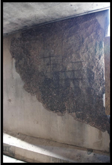
Figure 2.24 Fire spalling of the external wall of a garage. The heat source was three burning vehicles. Note the absence of spalling on the roof slab. The reason for the difference could be caused by (i) differences in concrete quality and/or (ii) difference in load situation where the wall element is loaded in compression. Photo Robert Jansson.
