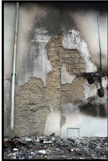
Figure 2.22 Fire spalling on an external concrete wall. The heat source was a burning tractor. Photo Robert Jansson.
