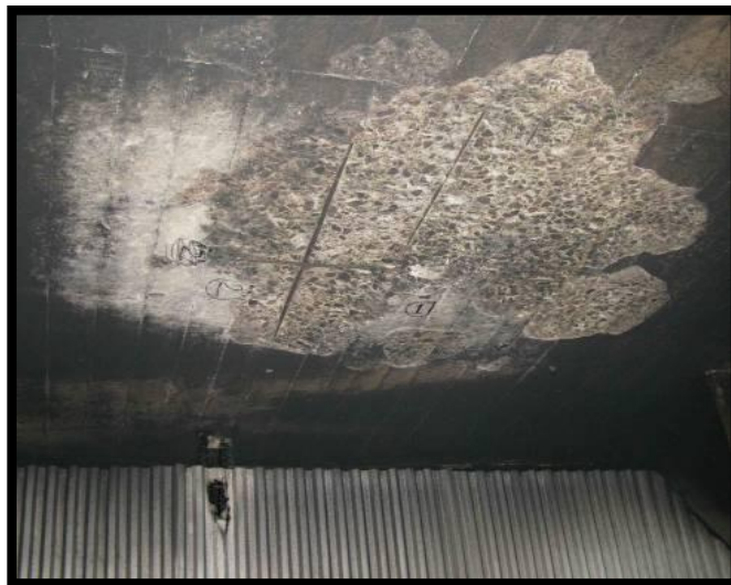
Figure 2.23 Fire spalling in the roof in a garage. The heat source was a burning car. Photo Robert Jansson.
